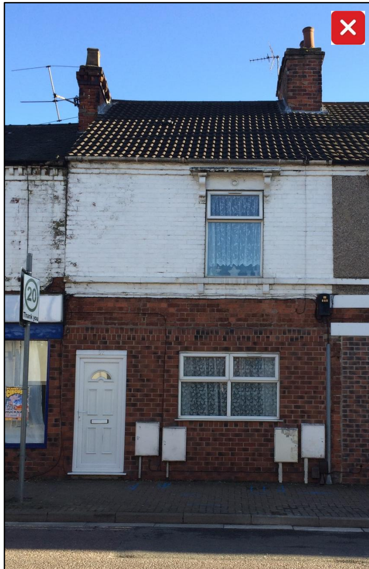
Poorly sited and designed meter boxes can spoil the appearance of the street and the property its self.
